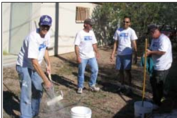
left to right: Quintus Schulzke (Project Leader), Eric McGar, Nikhil Khandelwal and John Ain clean up after rescuing the LVT roof.
